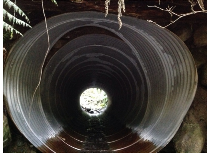
crushing and separating outlet
